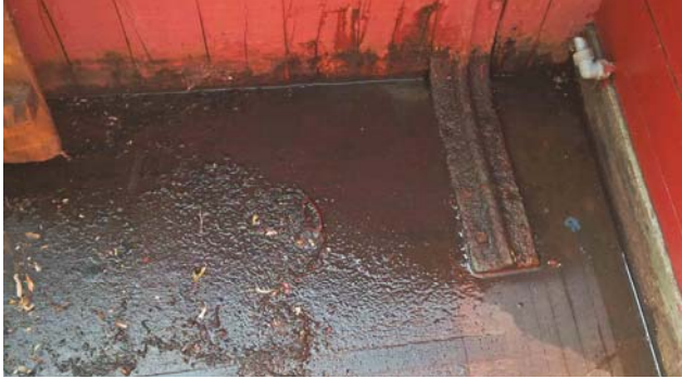
Signs of a probable leak, 28 June 2018.
