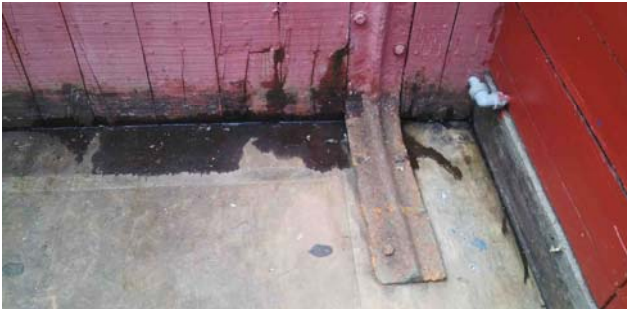
Evidence of the leak – note trickle of water on the right, 19 July 2018
