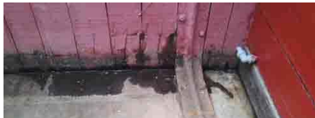
Evidence of the leak, 20 July 2018
