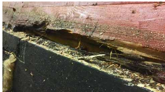
Rot in Raymond's cabin side, December 2016 Picture: Jem Bates
